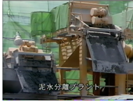
mud slurry separation plant
